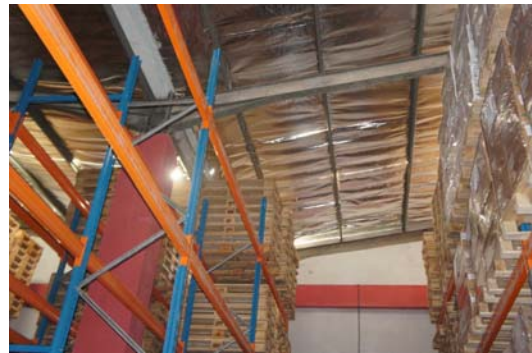
Rack installation around pillars & insulation appears to be damaged by excessive heat
