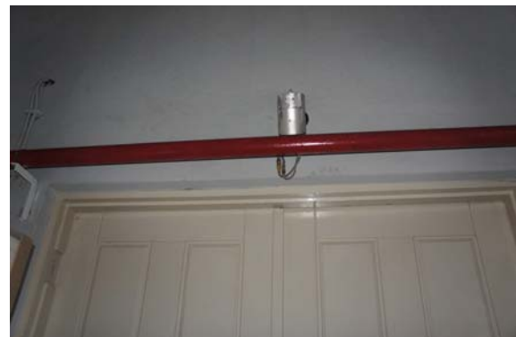
One of the non – functional CCTV cameras mounted in the MISAU warehouse
