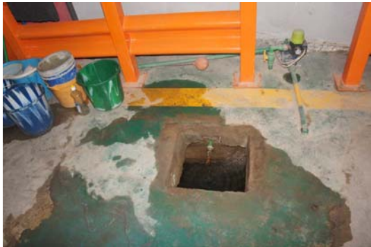
Water reservoir constructed under the floor of the Regional Warehouse in Nampula
