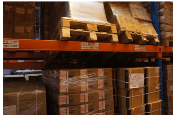
Collapsed beam of the Zimpeto warehouse rack system
